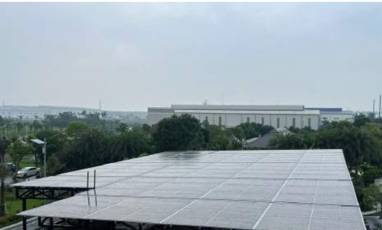
Solar power has been implemented
