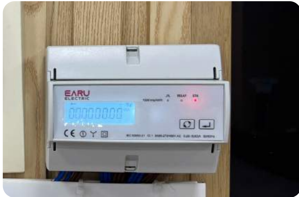
Continuous monitoring of total actual electricity consumption
