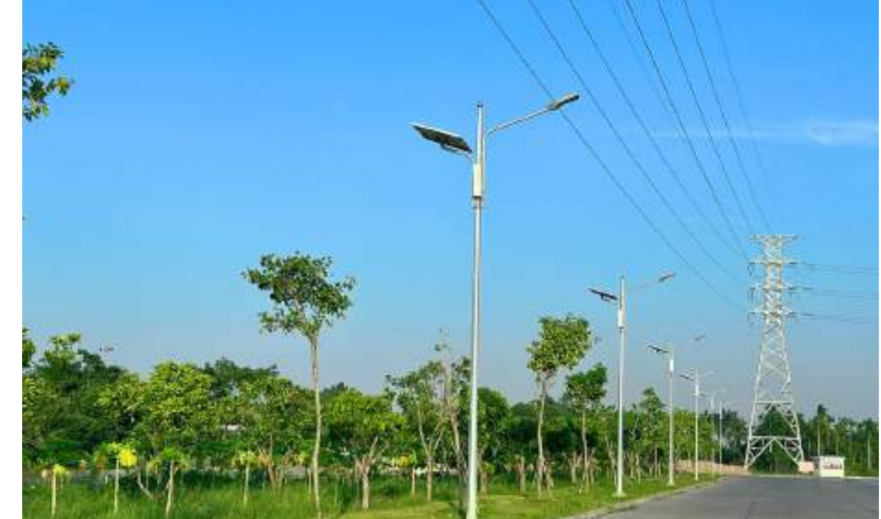
Solar power has been implemented.
